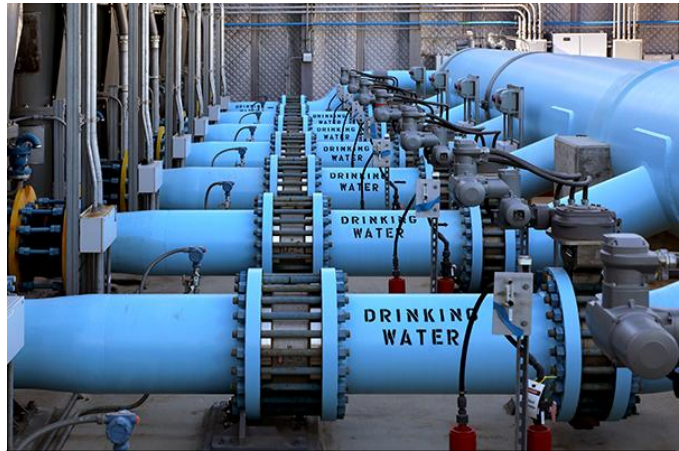
Claude “Bud” Lewis Carlsbad Desalination Plant, San Diego County Water Authority
